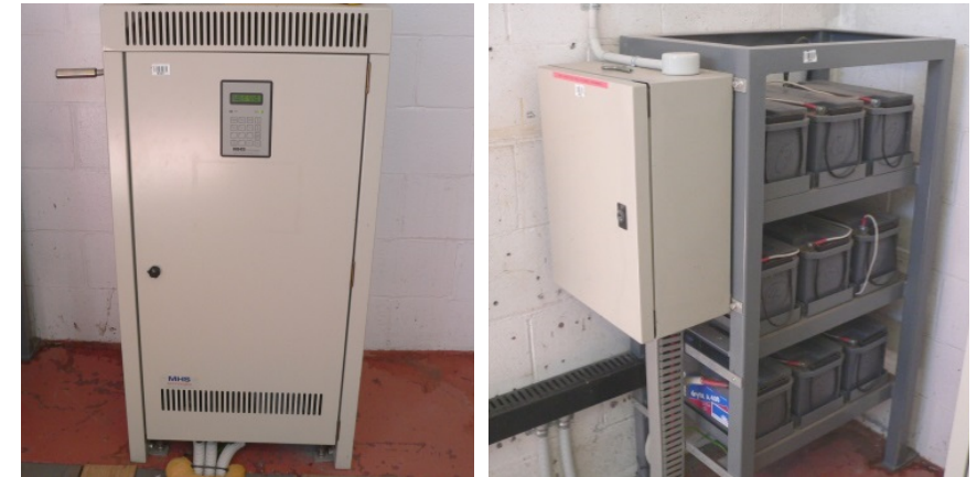
Figure 21.6: DC charger and battery bank
