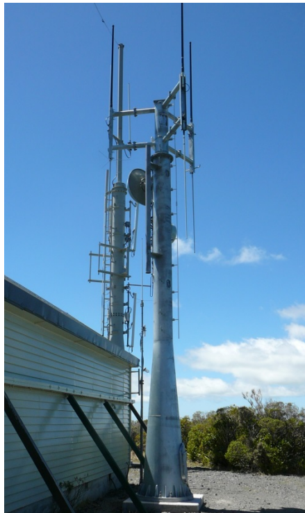
Figure 21.2: Communications mast with associated radio antennae
