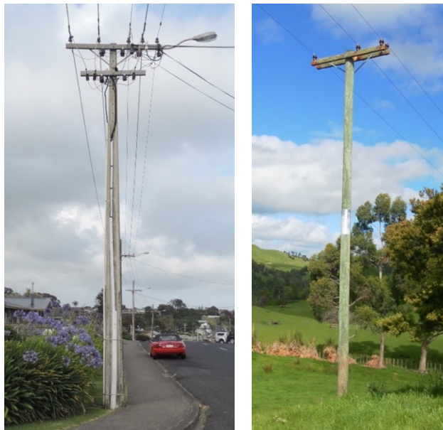
Figure 15.1: A modern pre-stressed concrete pole and a rural softwood pole
