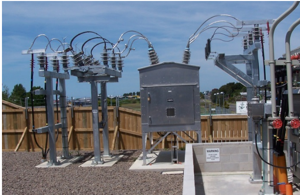
Figure 18.9: Typical outdoor 33kV switchgear bay
