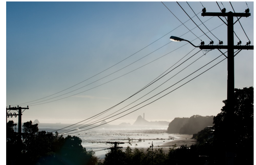
Figure 16.6: Distribution overhead line with LV underbuilt
