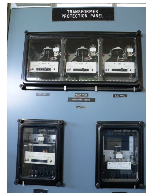
Figure 21.3: Electromechanical relays providing transformer protection
