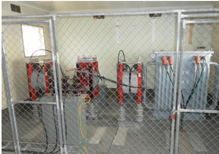
Figure 18.16: Load control injection plant
