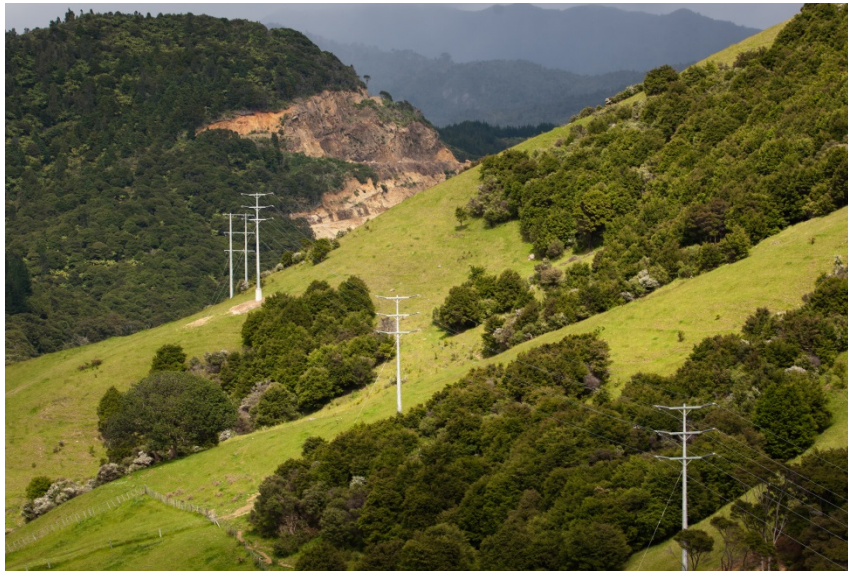
Figure 16.1: 66kV subtransmission overhead line in the Coromandel
