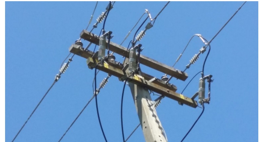
Figure 20.6: Pole-mounted drop out fuse
