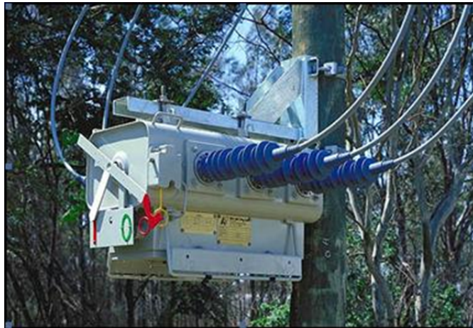
Figure 20.15: A pole-mounted sectionaliser
