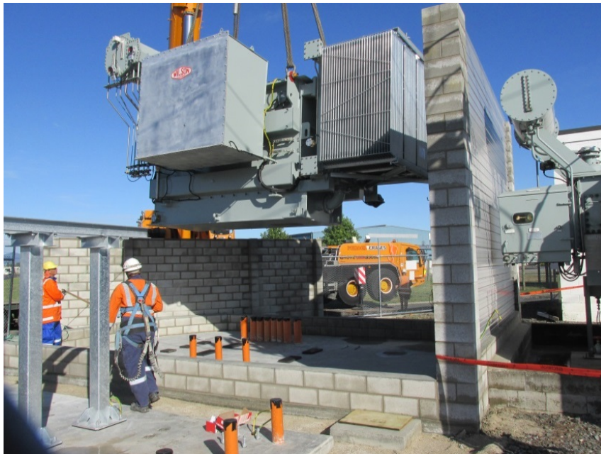
Figure 18.1: Power transformer installation at Waharoa
