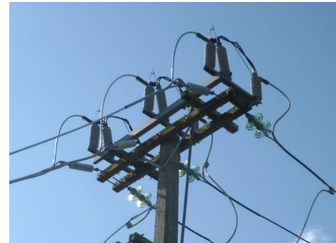
Figure 20.11: Air break switch (ABS)
