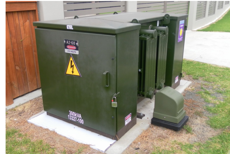
Figure 19.6: 300 kVA ground-mounted transformer
