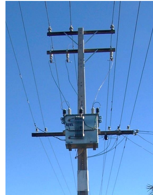
Figure 19.1: 100kVA pole-mounted transformer
