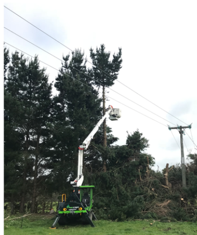
A tracked all-terrain EWP (elevated work platform) allows easy access to trees as well as minimising the impact on surrounding land.
