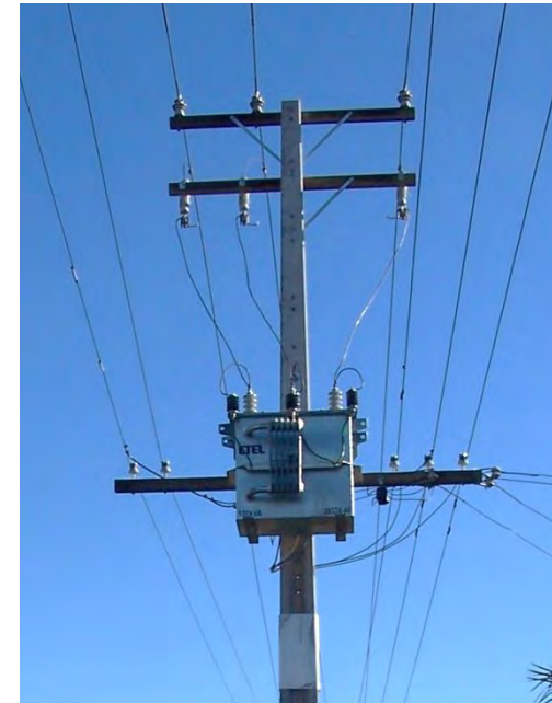
Figure 22.1: 100kVA pole-mounted transformer
