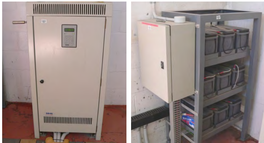
Figure 24.6: DC charger and battery bank
