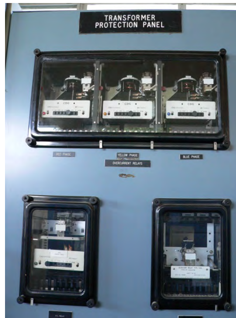
Figure 24.3: Electromechanical relays providing transformer protection
