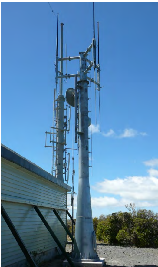
Figure 24.2: Communications mast with associated radio antennae
