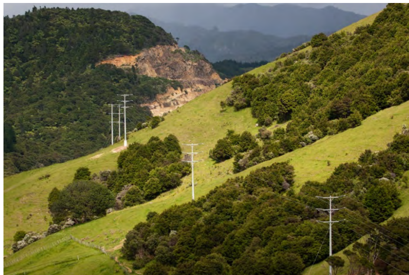
Figure 19.1: 66kV subtransmission overhead line in the Coromandel
