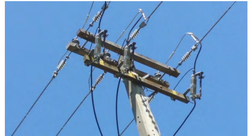
Figure 23.5: Pole-mounted drop out fuse
