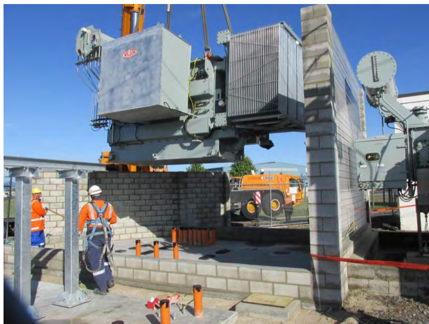
Figure 21.1: Power transformer installation at Waharoa
