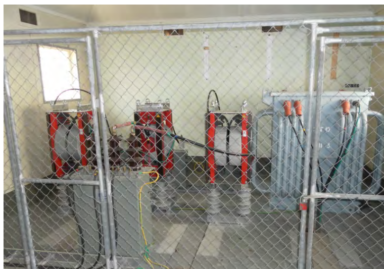
Figure 21.14: Load control injection plant
