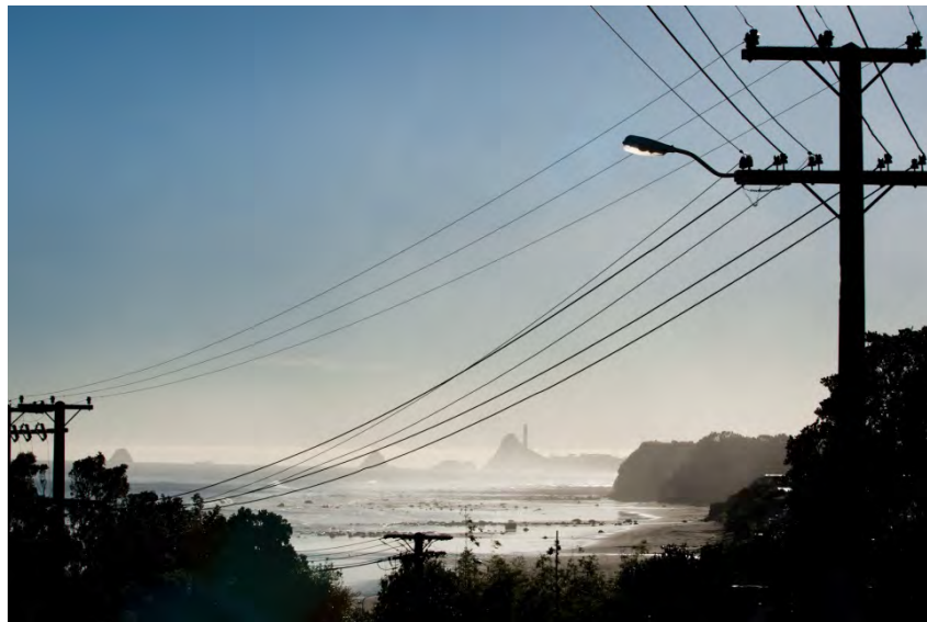
Figure 19.4: Distribution overhead line with LV underbuilt
